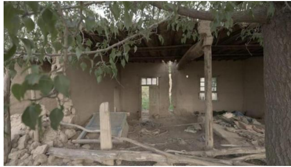
Figure 11 Collapsed Rammed-Earth House in Shangrun Village
